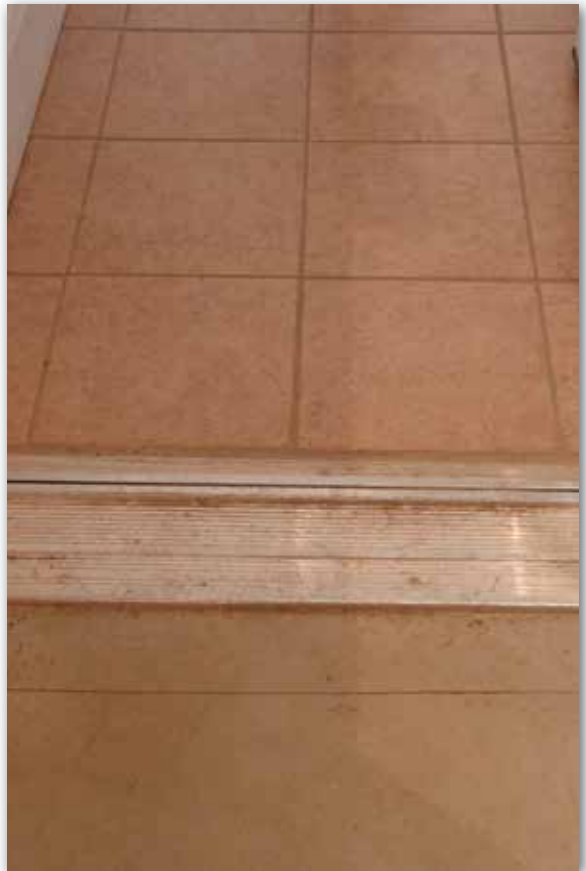
Use of an uncoupling membrane prevented this shrinkage crack (exposed in the mechanical room) from transferring through the tile and grout in the public areas of the showroom.
